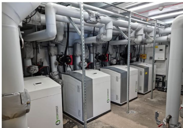
Site plant room
