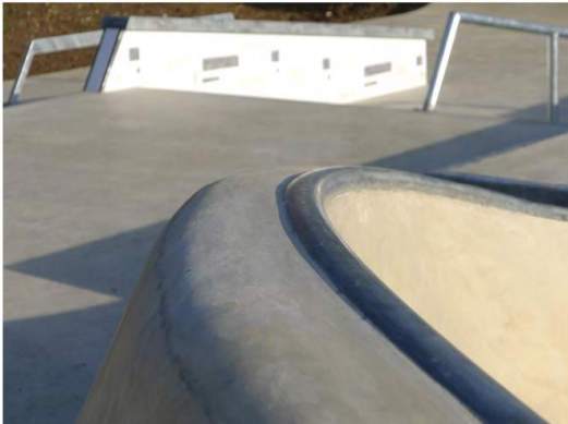
SKATEABLE EDGING IS PROTECTED WITH GALVANISED STEEL EDGING. THIS IS TO AID THE FORM'S USE IN TANDEM WITH CREATING A PROTECTED EDGE.
